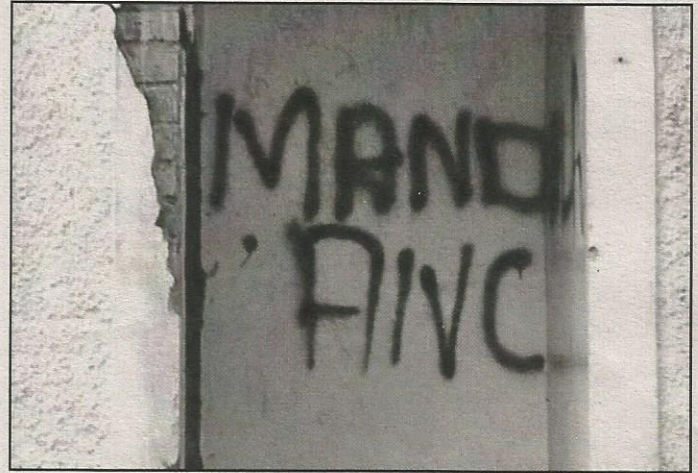
Slogans were sprayed on the walls of dressing rooms. Photo: Alex van Rensburg
